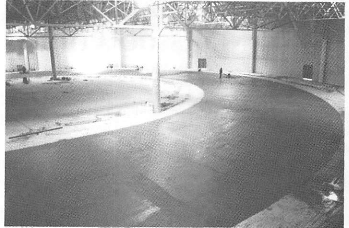
The figure in the middle of the turn is machine troweling the surface. This gives an idea of the massiveness of the track.
